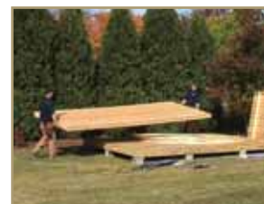
Sections are carried to site and floor is leveled on concrete blocks
